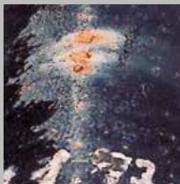
Non-zinc coated: the damage is worsened and the corrosion (red marks) extends beyond the notch
